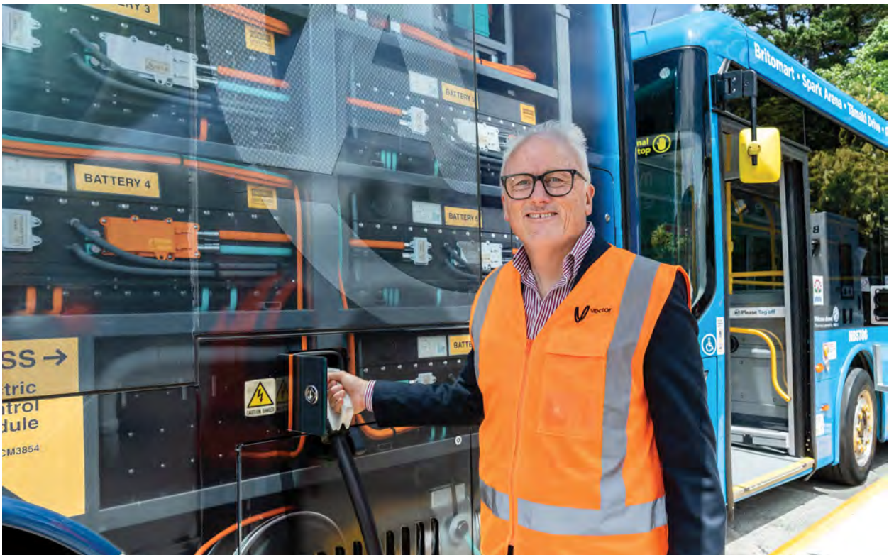
Launch of New Zealand's first fully electric bus depot with the capacity to charge 20 - 30 buses each. Charging at this depot occurs within a 'dynamic operating envelope', where Vector forecasts optimal charging times each day and provides this through to the depot, reducing peak demand for a more affordable charging solution.
