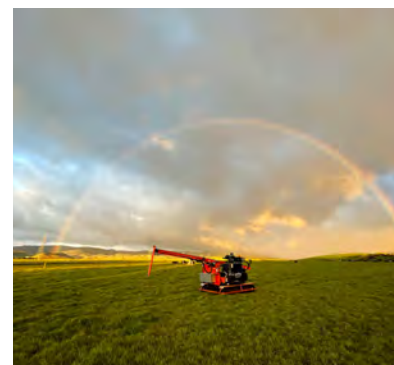
Thor, one of Vector Powersmart's GAYK machines that can drive piles into the ground twice as fast as traditional methods for faster assembly of large-scale ground-mounted solar farms.
