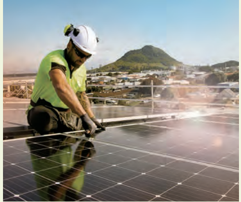
— INSTALLATION OF ONE OF POWERSMART'S PROJECTS, AT THE NEW ZESPRI HQ IN MOUNT MAUNGANUI.
