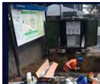
Mobile transformers have been successfully trialled as an alternative to diesel generation
